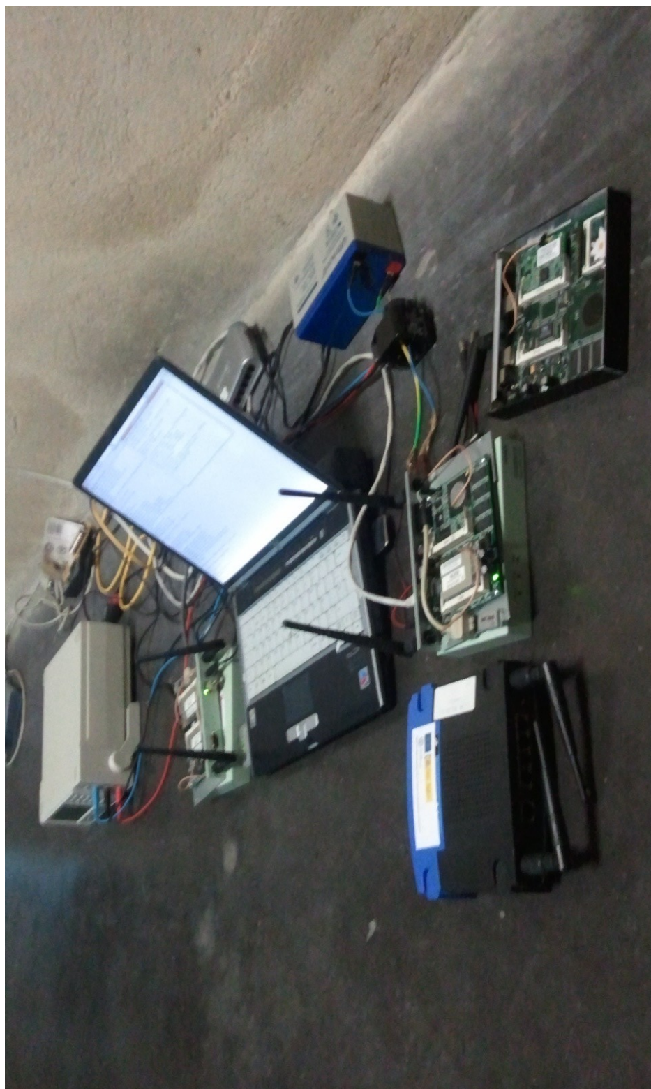
Figure 7: Picture of the deployed testbed.
